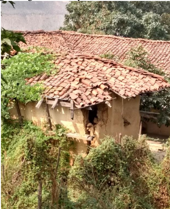
Figure 33 Household in lat which has been destroyed due to blasting in the Chhal Open Cast Coal Mine
